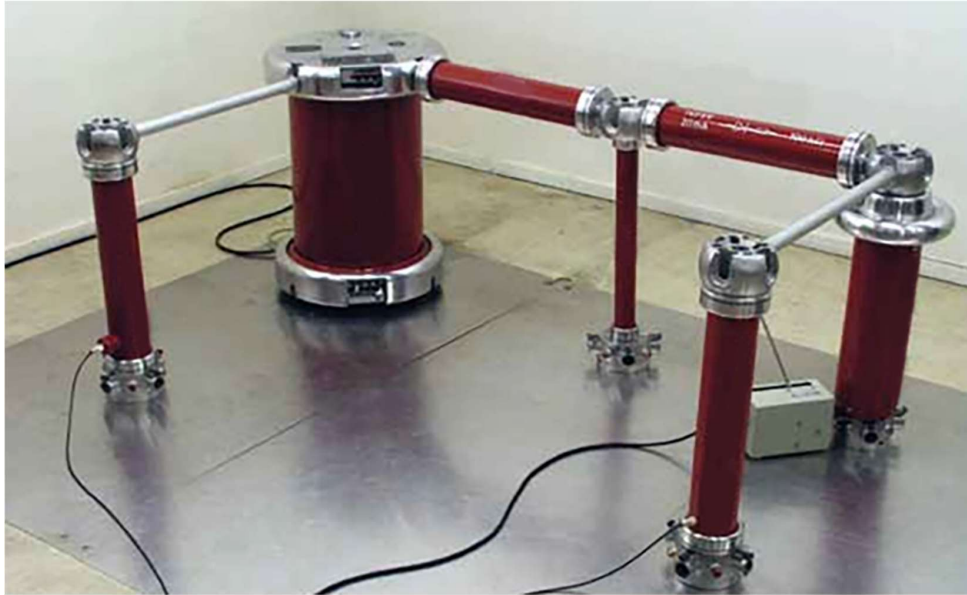
Single-stage DC Voltage Test Set-up (In the picture above AC-divider + Connecting Rod incl.)
